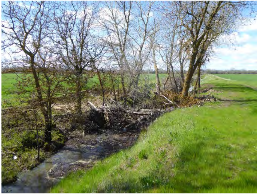
Debris obstruction along northern irrigation canal
